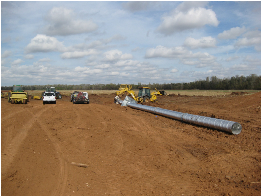
The photo is taken in the Big Bottom Unit and is the installation of the new drainage structure to allow for the manipulation of water. Lots more work will occur in 2011!
